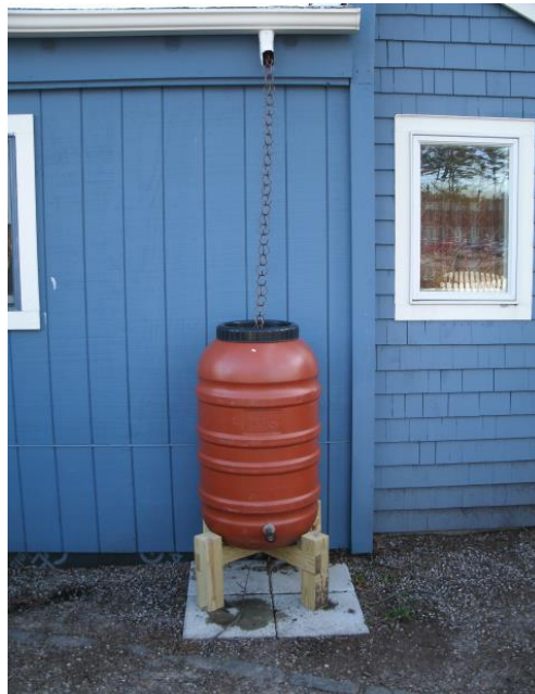
Rain barrel BMP installed at Bobs Clam Hut, Kittery, Maine
