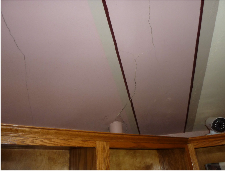
Photo 7: Second floor plaster ceiling. Note the cracks in the plaster.
