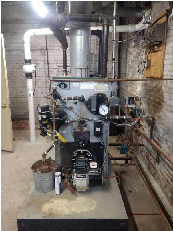
Figure 5 – Oil Fired Boiler
