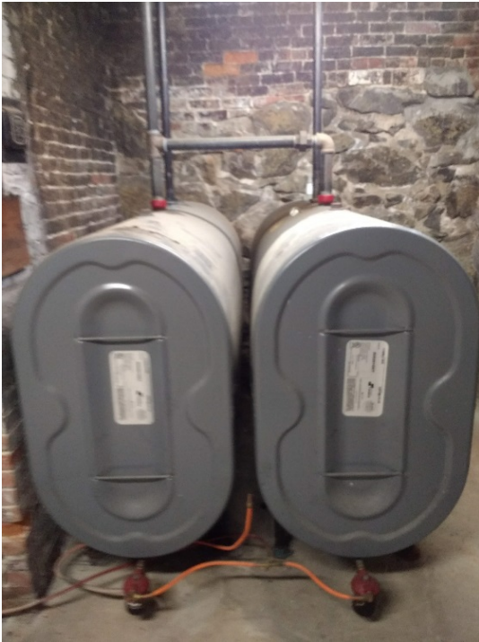
Figure 3 – Oil Storage Tanks
