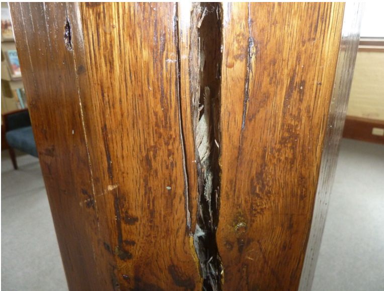
Photo 6: octagon wood column in basement. Note the large checks.
