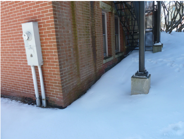
Photo 8: North east corner of building. Note the dirt below the fire escape and some minor effervescence at the base of the wall.
