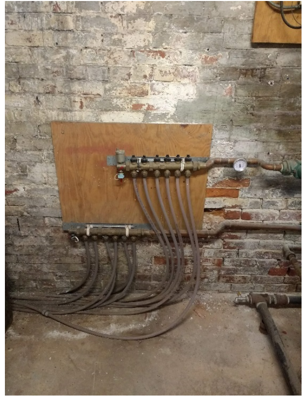
Figure 6 - Radiant Floor Manifolds
