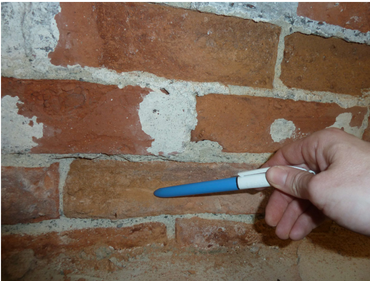
Photo 2: Basement boiler room. Close up of soft brick.
