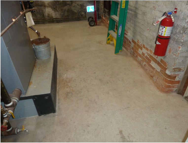
Photo 1: Basement boiler room.
