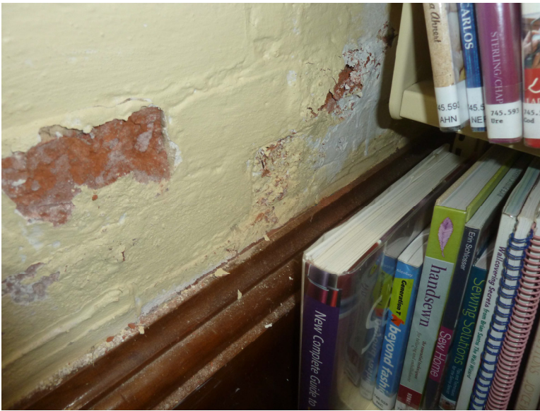
Photo 4: Basement reading room. Close up of exterior wall showing paint and brick damage.
