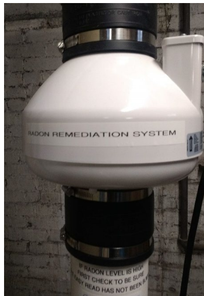
Figure 9 - Radon Mitigation System
