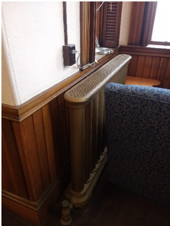
Figure 10 – Typical Radiator on Second Floor
