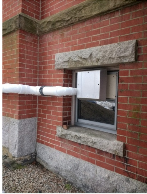
Figure 8 - Boiler Combustion Air Supply Fan Intake
