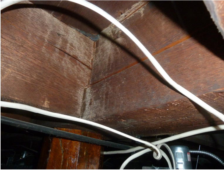
Photo 5: first-floor framing showing wood column, girder and wood joist. Note the horizontal split in the wood girder.
