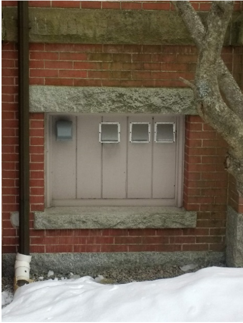
Figure 7 – Bath Fan Exhaust Hoods
