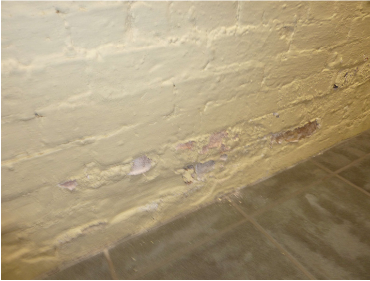
Photo 3: Kitchen area. Close up of interior wall showing paint and brick damage.
