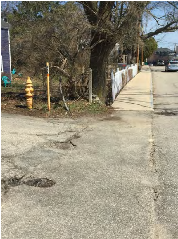
Lack of crosswalks for side streets and ADA compliance.
