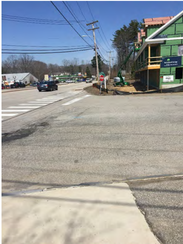
Sidewalk ends and ADA compliance.
