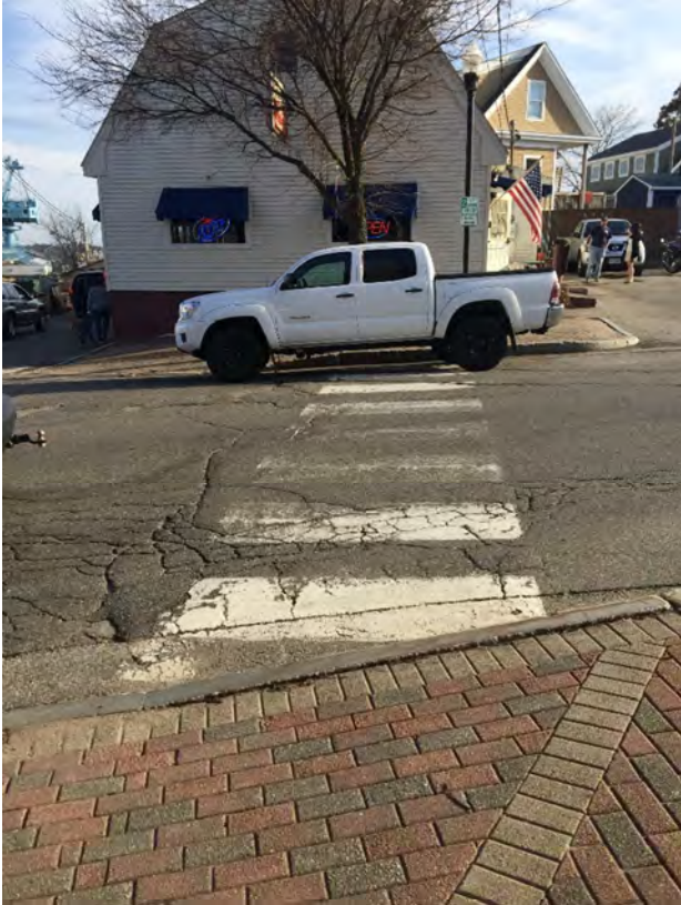
Crosswalk is not oriented with the ramp
