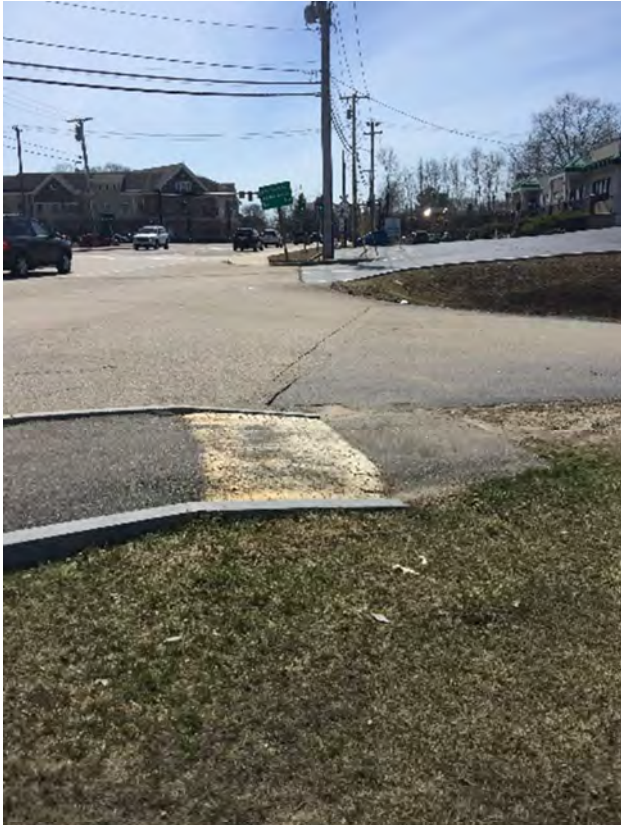
ADA compliance and lack of crosswalk markings.
