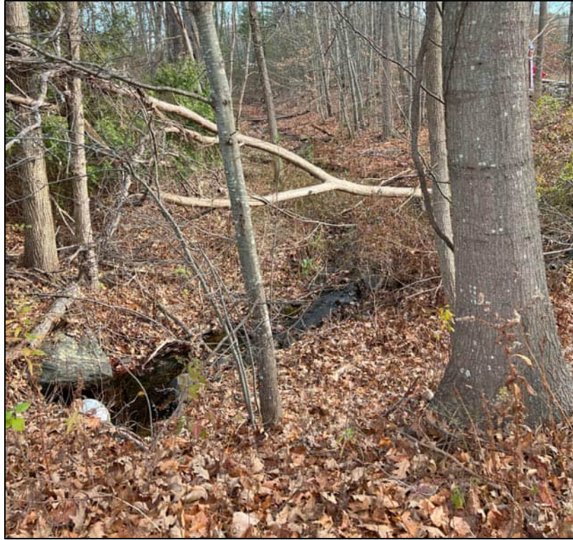
Drainage channel conveying drainage from area north of Martin Road (DA-1-1) toward Highway 236 (CB-1-3).
