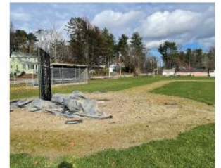
Photo 6: Batter's circle and base lines in fair condition, evidence of ponding and moss growing.
