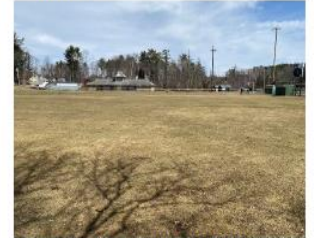
Photo 2: Dips and heaves in right field.
