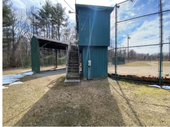
Photo 8: The press box at the backstop is not ADA accessible, with bare spots and evidence of ponding.
