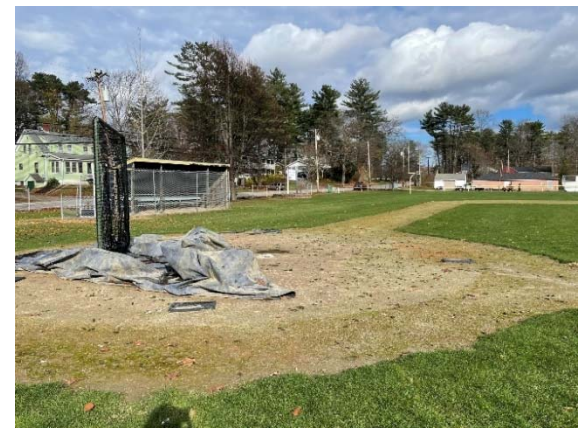
Photo 6: The batter's circle and base lines are in fair condition, with evidence of ponding and moss growing.
