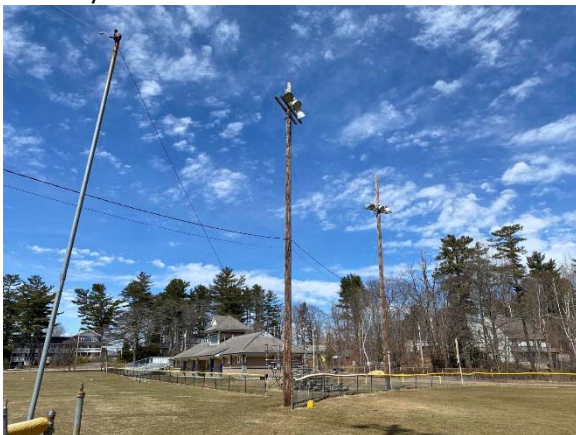
Photo 3: Athletic lighting fixtures and poles are outdated and in fair condition.
