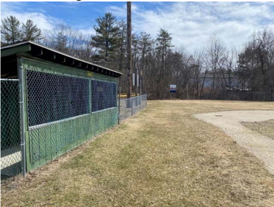
Photo 3: The dugout is in fair condition; the fencing on the dugout frayed at the bottom and there is evidence of ponding.
