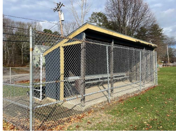
Photo 8: The left field dugout is in fair condition, is not ADA accessible, and shows evidence of ponding.
