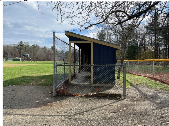
Photo 10: The right field dugout is not ADA accessible, and has bare spots and evidence of ponding.
