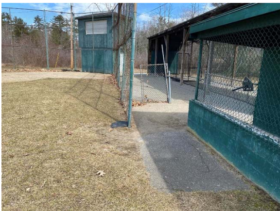
Photo 5: The dugout, backstop, and site fencing are in fair to poor condition. There is evidence of ponding at the dugout.
