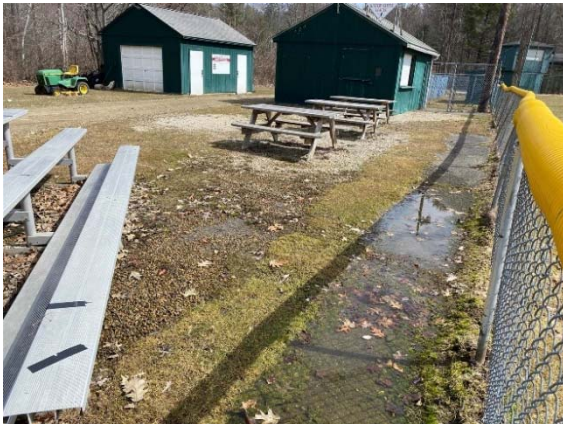
Photo 11: The spectator seating area has many bare spots and evidence of significant ponding.
