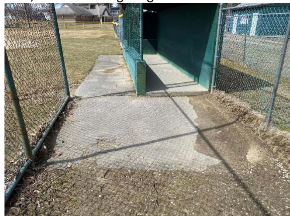
Photo 6: The dugout is not ADA compliant and significant ponding appears to occur at the dugout.
