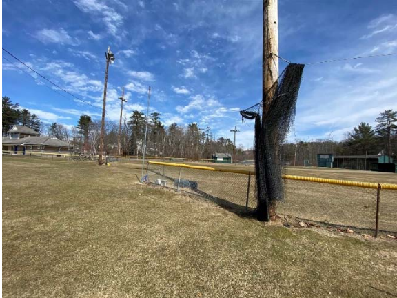
Photo 1: Safety netting appears to be ripped and currently not in use.
