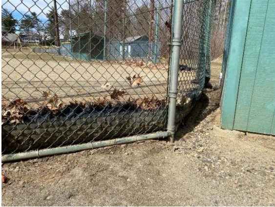
Photo 7: There is a significant elevation change at the backstop and evidence of erosion and sedimentation.
