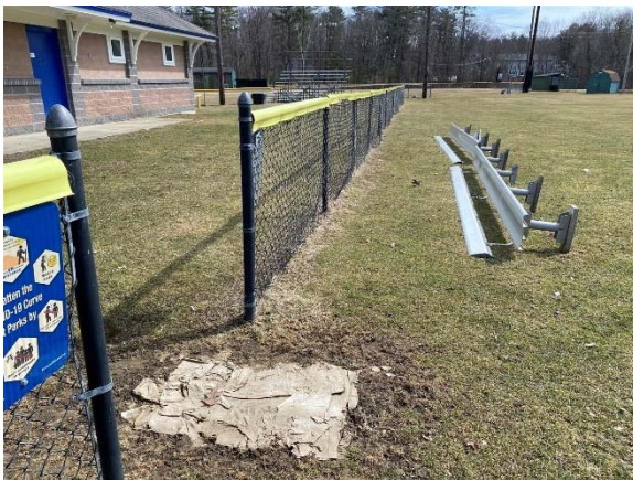
Photo 3: View of the football field benches and fencing in fair condition. There are signs of ponding along the football field fence.
