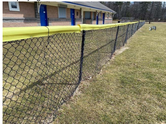
Photo 4: Football field fencing is in fair condition. There are signs of ponding along the fence.
