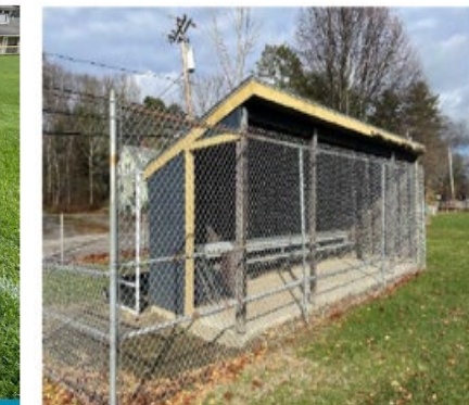
Photo 8: The left field dugout is in fair condition, is not ADA accessible, and shows evidence of ponding.
