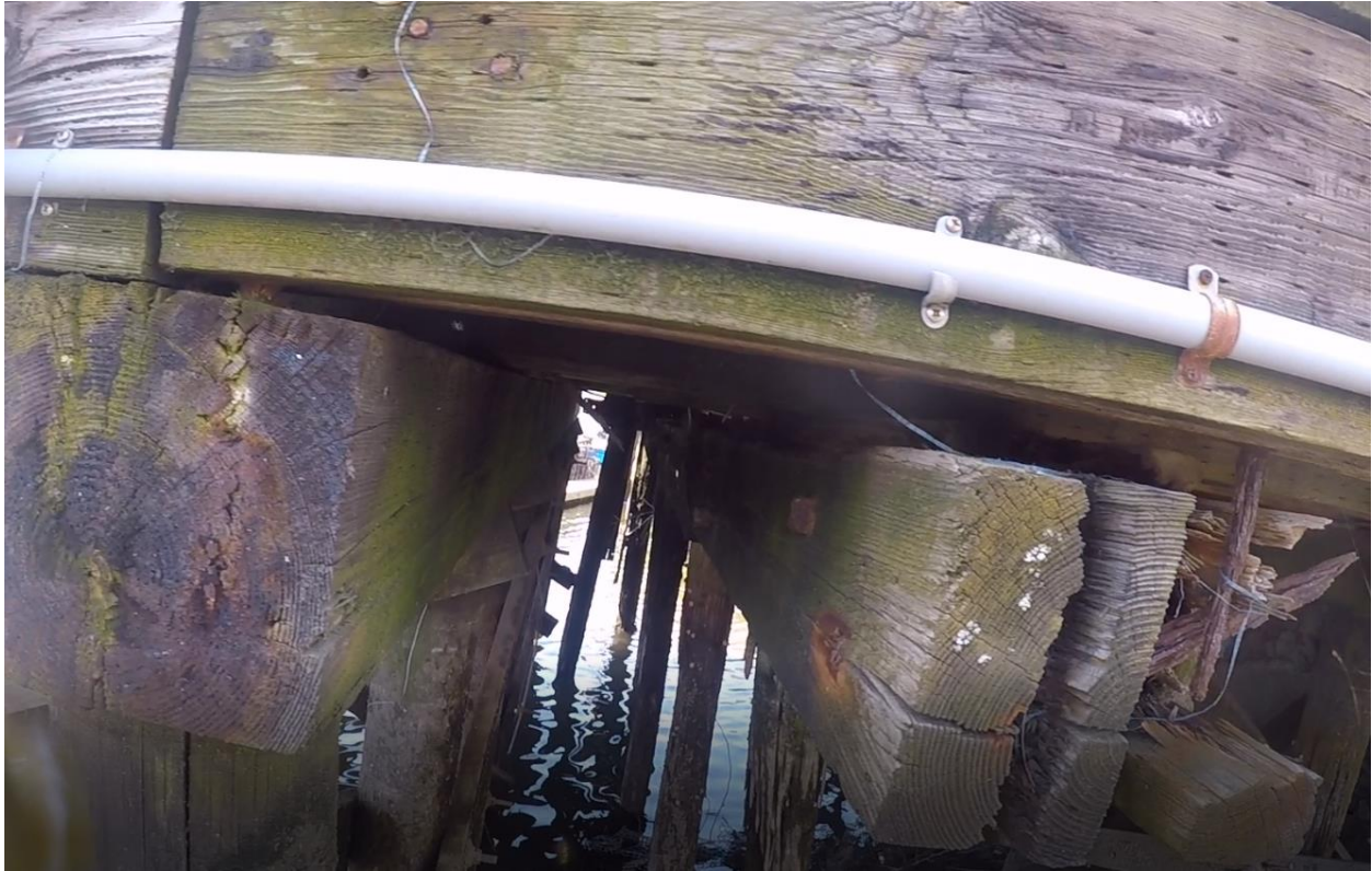
Figure 32 – View of Pier framing on east edge. Note: outer stringer lifted due to hoist tension anchor.
