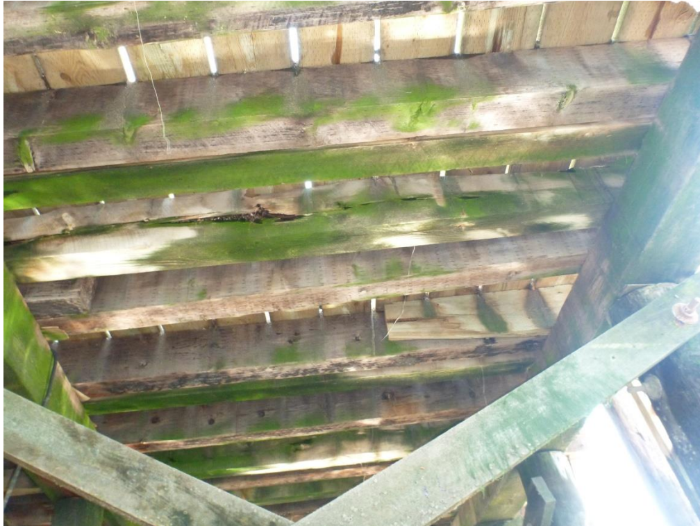
Figure 14 – Pier Stringers (Note: more algae growth and visible rot on older stringers)
