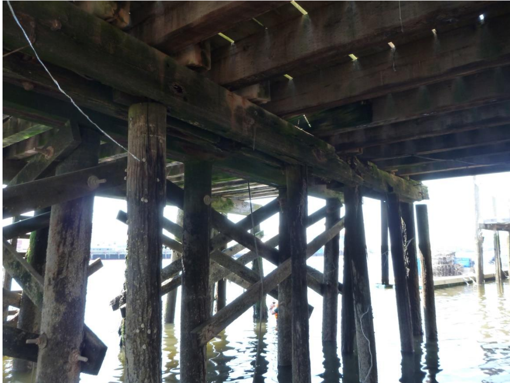
Figure 20 – View of Bent 3 in very poor condition (believed to be abandoned)
