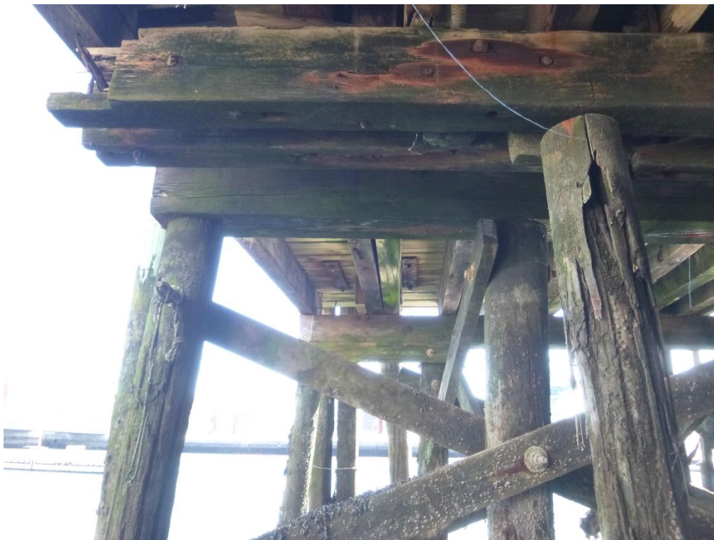
Figure 35 – Underside of southeast corner of pier, note: hoist only fastened to decking
