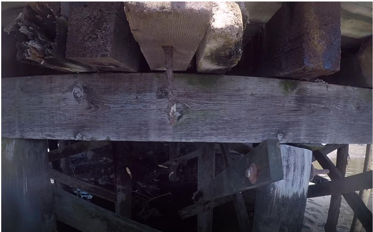
Figure 31 – View of Pier framing from water side, note: multiple generations of closely spaced stringers
