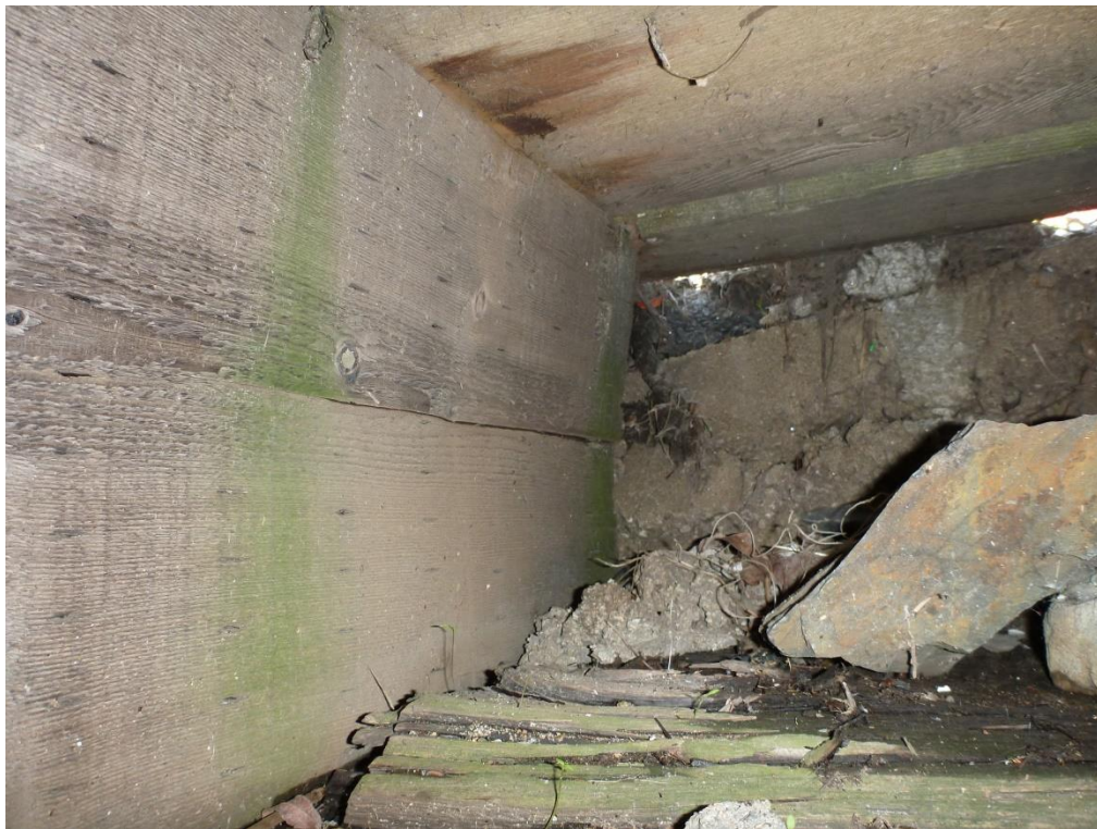
Figure 19 – Failure of stringer at Line 5
