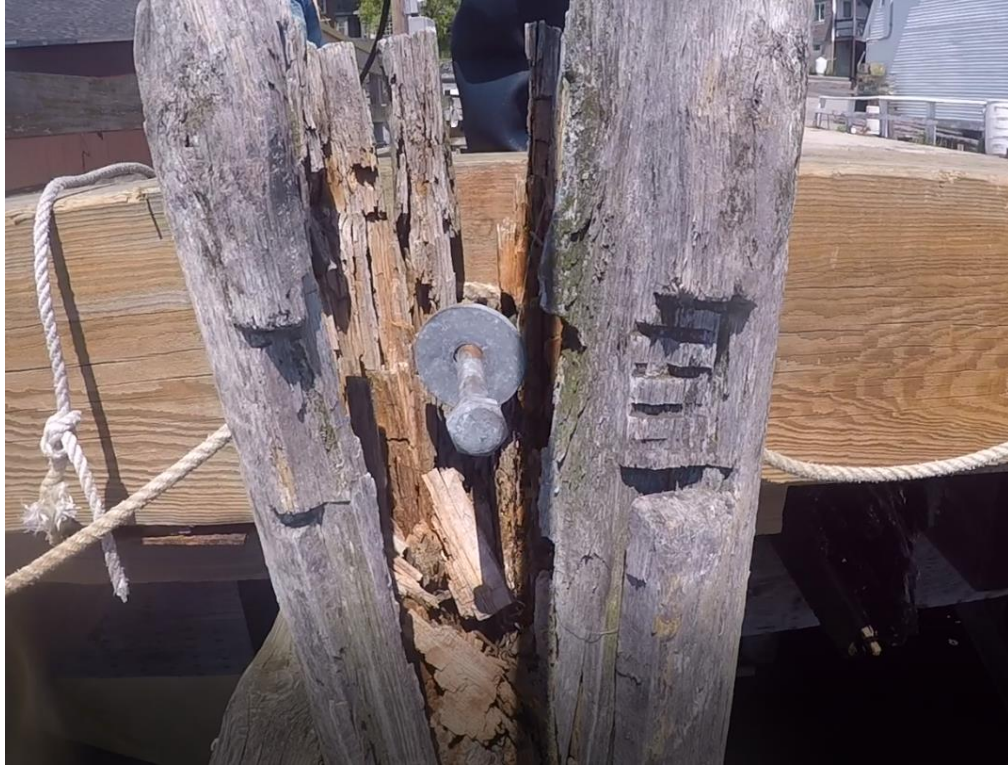
Figure 30 – Fender Pile Deterioration, view from water side
