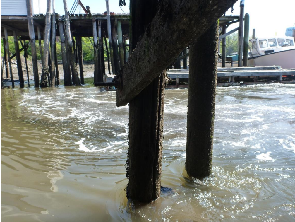
Figure 24 – End pile on Bent 4. Note: More severe deterioration
