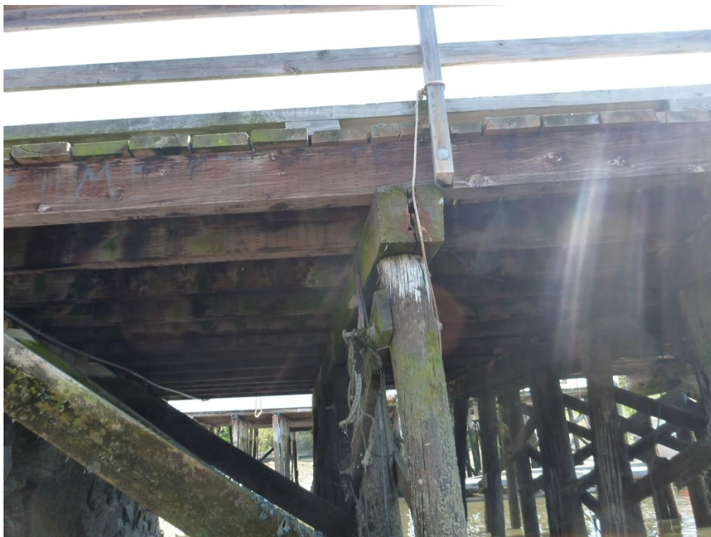
Figure 21 – West end of Bent 4. Note: Split in pile cap, striations in end pile
