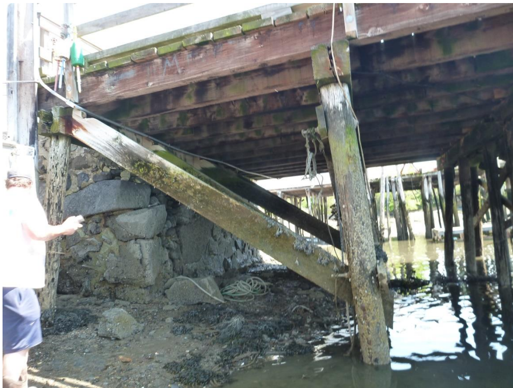
Figure 17 – West end of bents 4 & 5. Note: significant deterioration of pile caps 4 & 5
