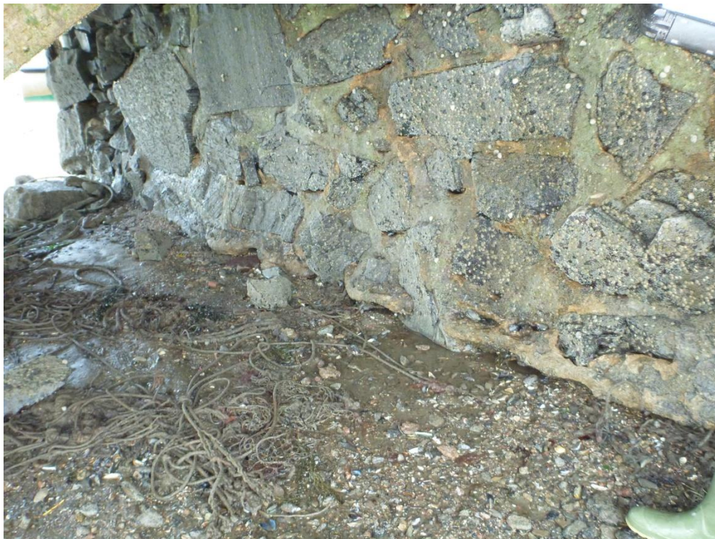
Figure 11 – Stone faced bulkhead. Note: water seepage beneath bulkhead
