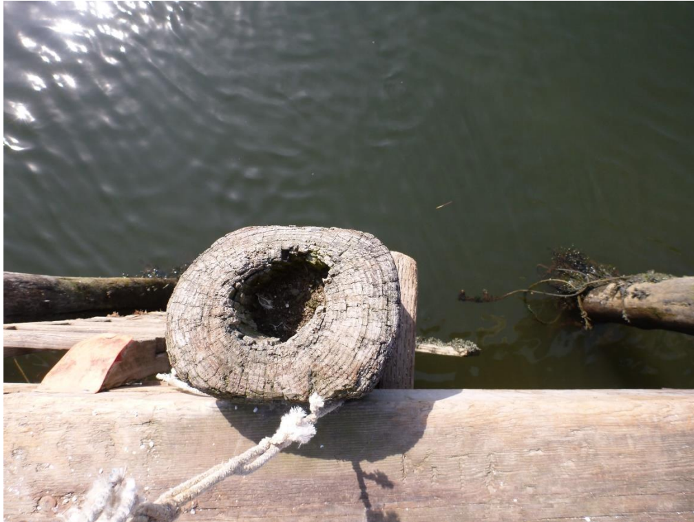
Figure 28 – Fender Pile at working face showing moderate rot
