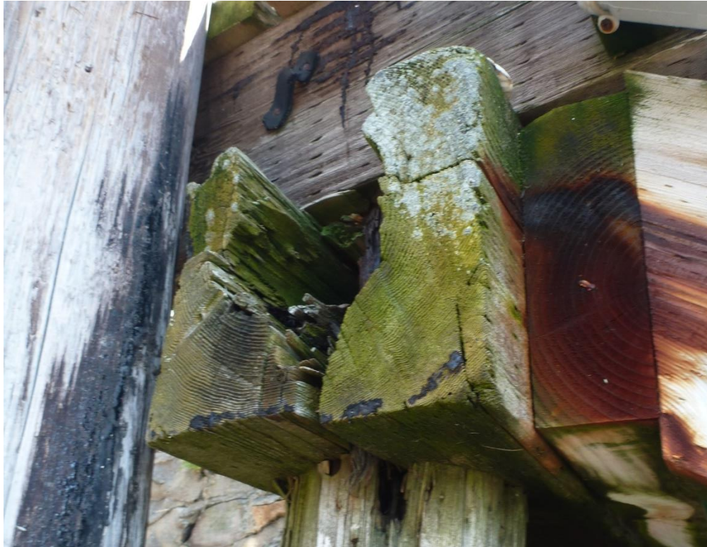
Figure 22 – West end of Bent 5 Pile Cap. Note: Near complete failure of pile cap, significant rot in pile
