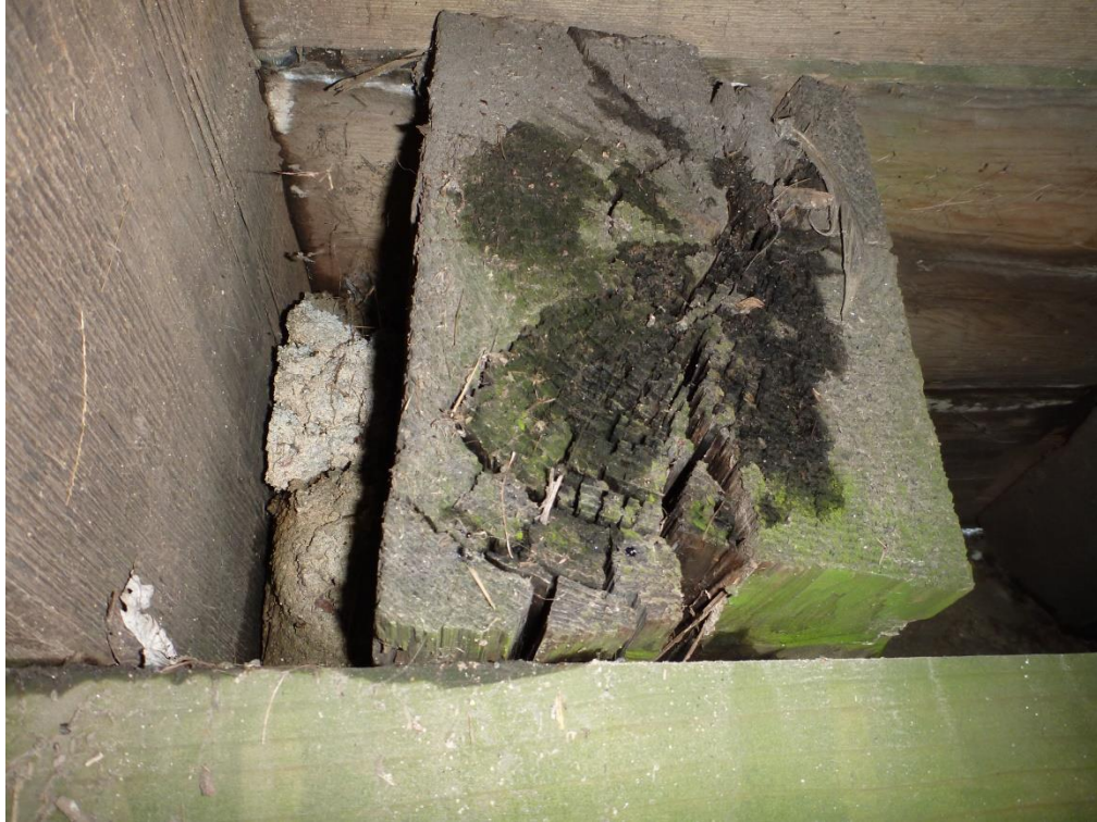
Figure 18 – Significant deterioration of stringer near Line 5
