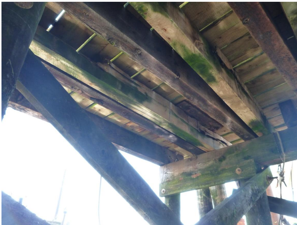
Figure 15 – Pier Stringers (Note: more algae growth and visible rot on older stringers)
