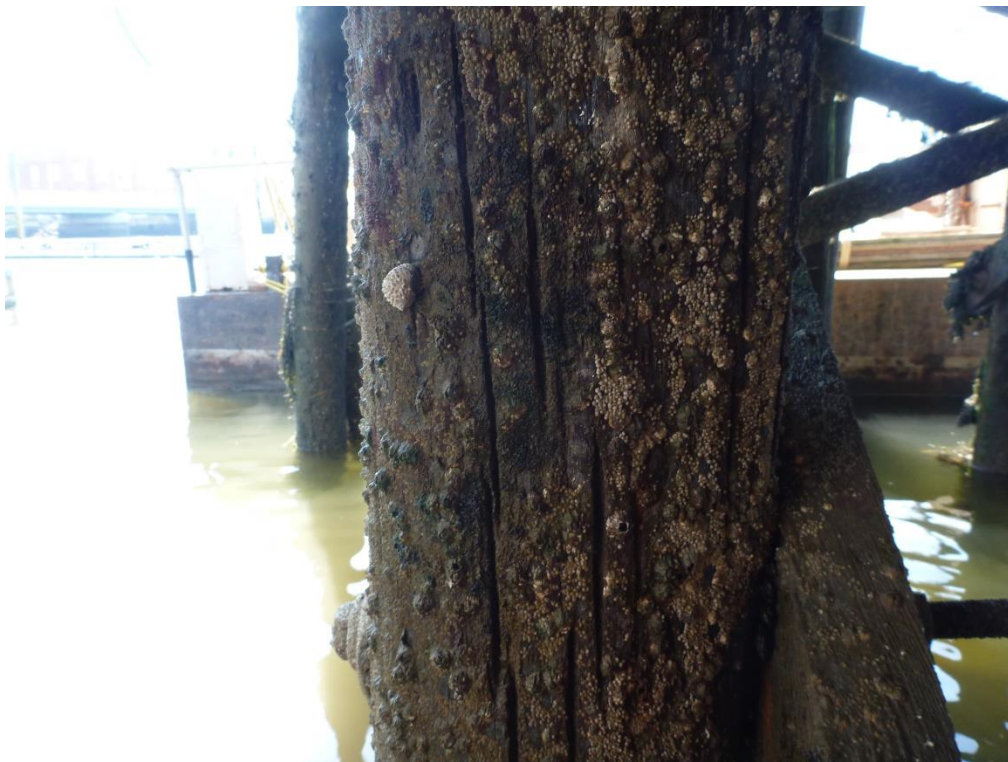
Figure 25 – End pile on Bent 4. Note: more severe deterioration
