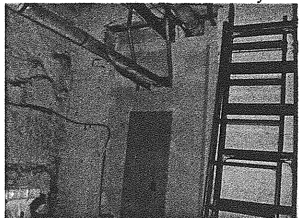
TSI intersect with Staff Bathroom wall in Mechanical Room of Public Library.
