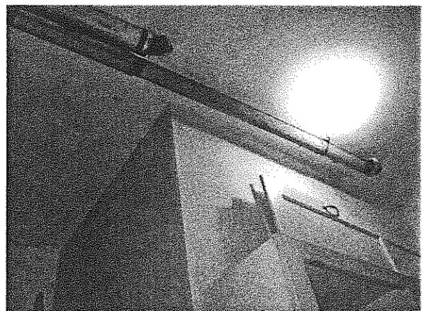
TSI on pipes in Mechanical Room of Public Library.
