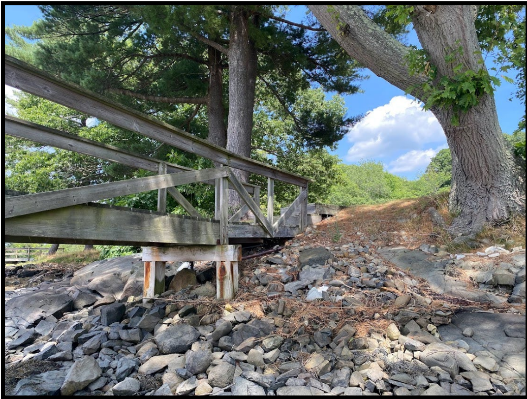
Photo 4: Existing Pier Structure Facing Northeast – Damaged Stringers
