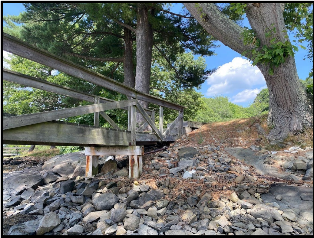
Photo 4: Existing Pier Structure Facing Northeast – Damaged Stringers
