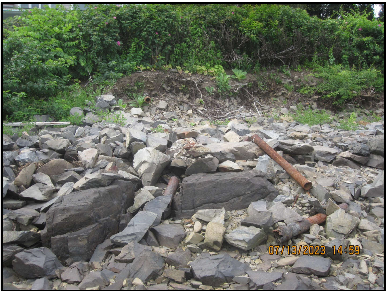
Photo 2: View showing exposed soils and root systems, shifted riprap, and a broken pipe (07/13/2023)
