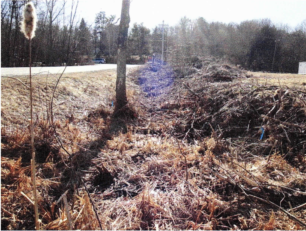
View Of The Wetland Area That Meets The Town of Kittery's Definition Of A Drainage Ditch
