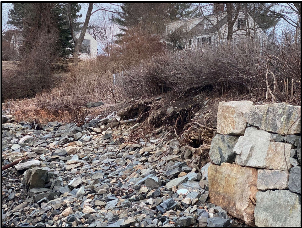
Photo 1: View showing slope failure, exposed soils, eroding vegetation, and exposed root systems (01/18/2023)
