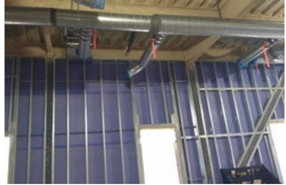
Figure 2: First Floor Duct Work
