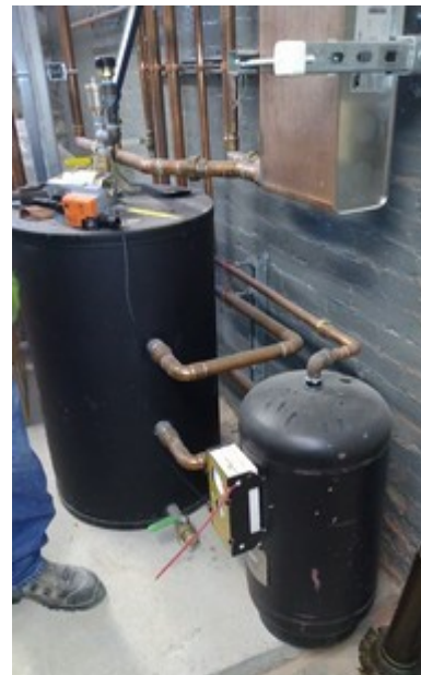
Figure 4: Boiler Room Buffer Tank & Heat Exchanger
