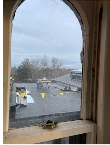
4. View of EPDM roof over the Children's Reading area and Children's Lobby.
