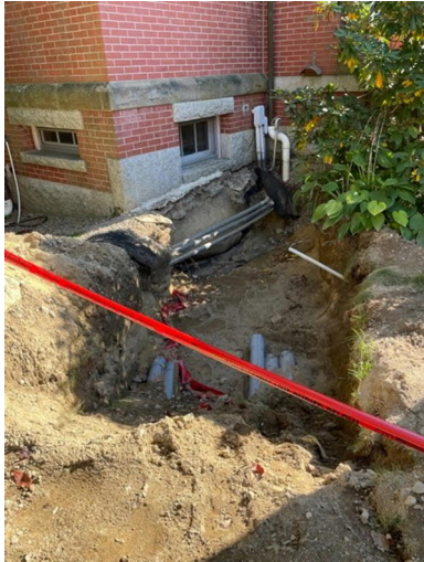
3. View of the electrical service to the building.
