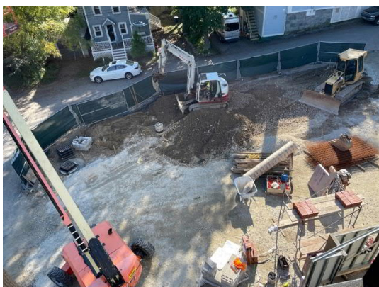
7. View from above looking down at new lower parking lot area being graded.
