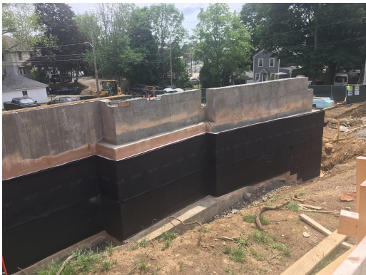
1. Northwest corner of addition: Insulation and waterproofing the foundation wall below new entrance.
