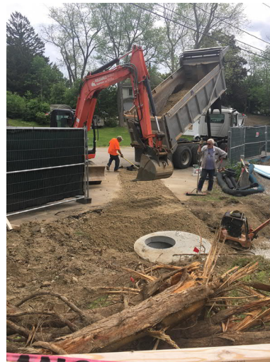
6. Southeast side: Install of catch basin by new addition and existing building.
