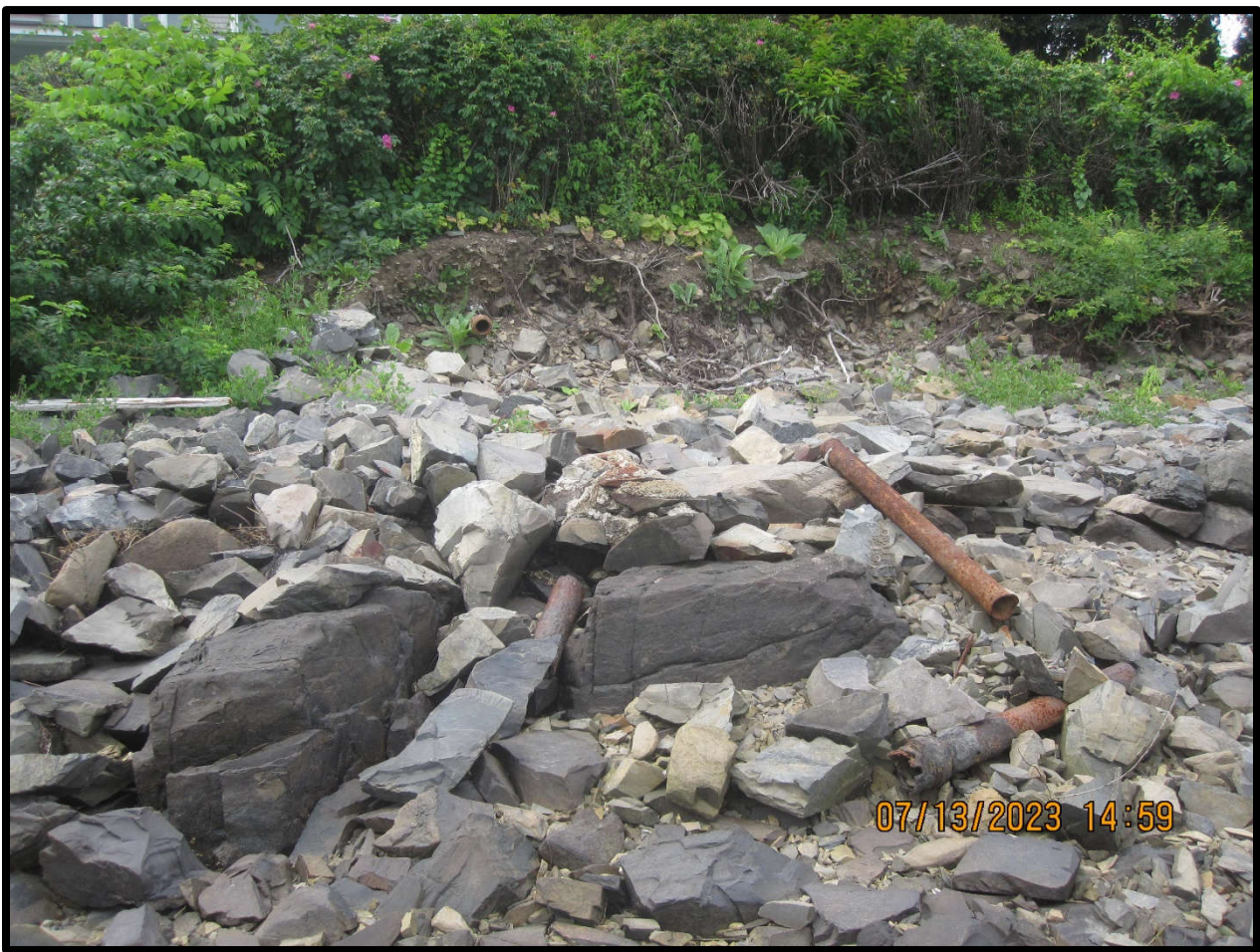
Photo 2: View showing exposed soils and root systems, shifted riprap, and a broken pipe (07/13/2023)
